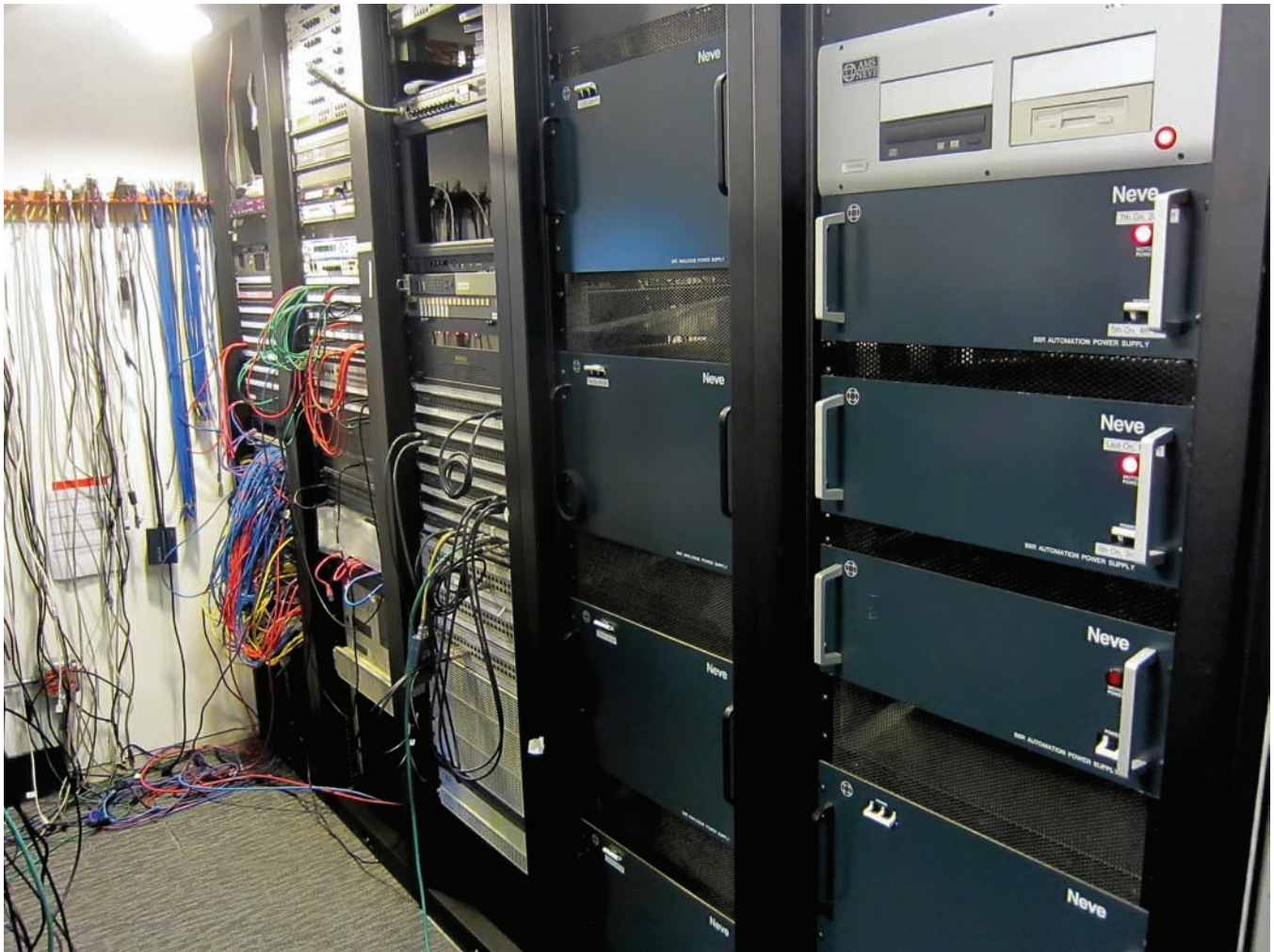
Fig. 9 Fox Scoring Stage Machine Room (right side).
