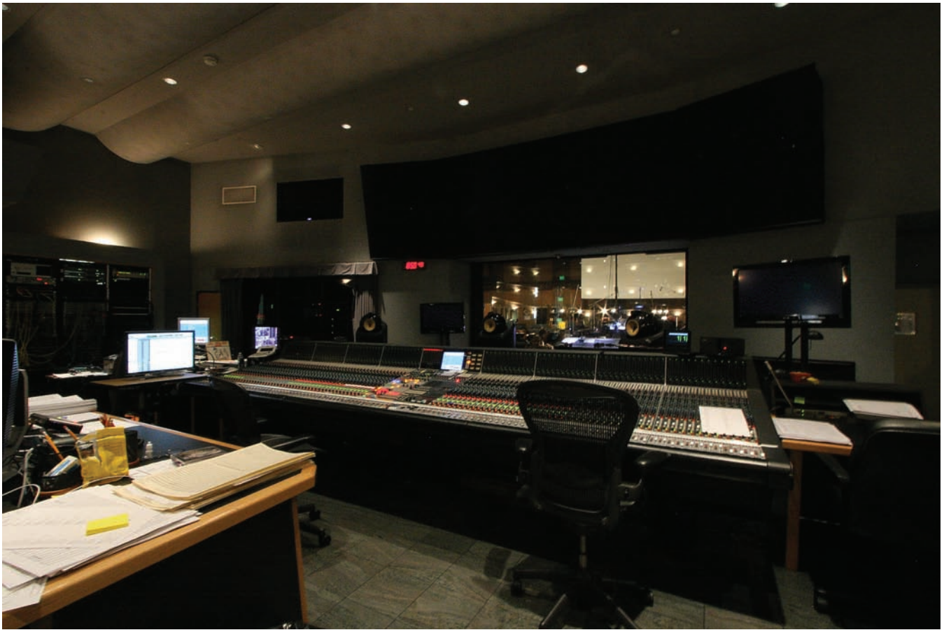
Fig. 4 Sony Pictures Control Room.
